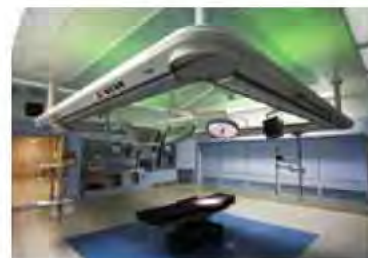
Operating Room OPERA System (Dräger)
